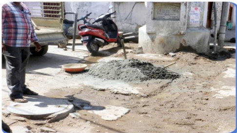
Unrepair Road at Masjid Circle Vemukunta (Before)
