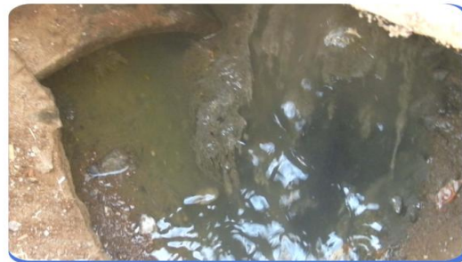
Manhole without cover at Vemukunta
