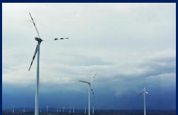
Brahmanvel Wind Farm: 528MW
