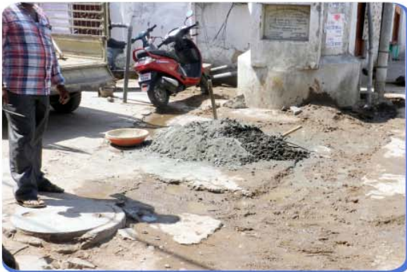
Unrepair Road at Masjid Circle Vemukunta (Before)
