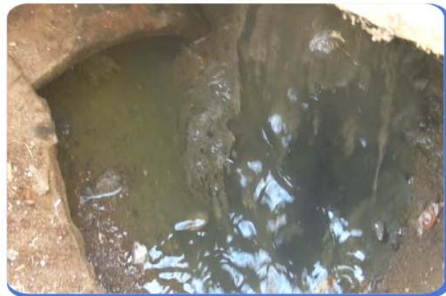
Manhole without cover at Vemukunta
